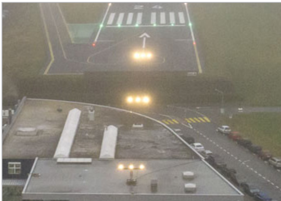
Fig. 4: APCH and RWY lights at Les Eplatures airport (LSGC) activated by the advanced ARCAL
